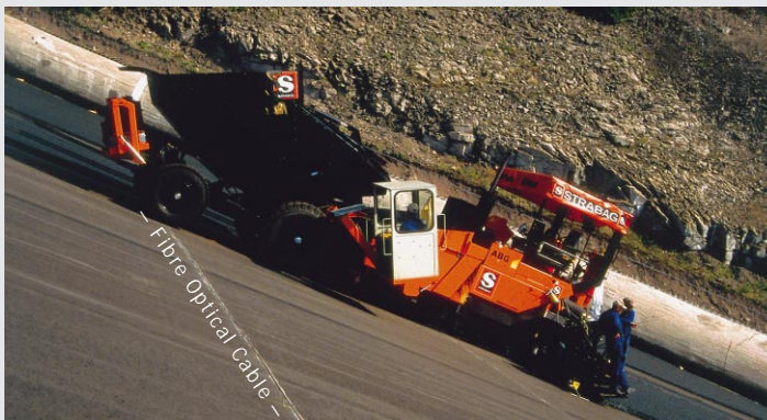
Installation of a hybrid fibre optical cable in the double layered asphaltic facing of the Ohratalsperrre, a rockfill dam in Thuringia, Germany, for leakage detection
