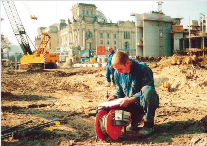
Leakage detection in a trough excavation pit in Berlin
